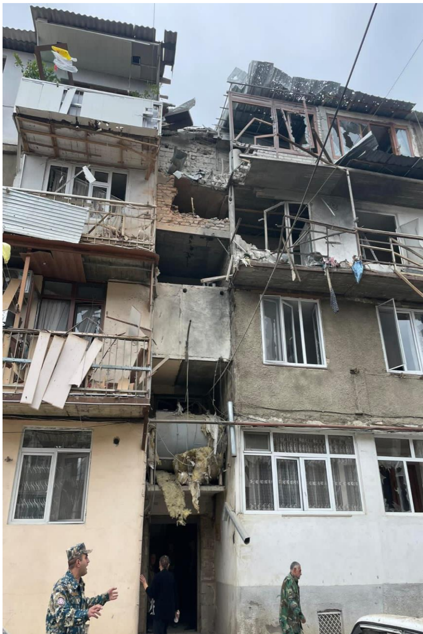
Damage to an apartment complex in central Stepanakert 183
